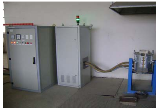
Fig.1. Induction heating furnace of medium frequency (8000 Hz).
