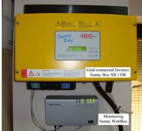
Fig. 4 Grid-connected inverter and monitoring system.
