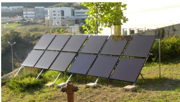
Fig. 3 Photograph of the 720 Wp solar PV power panels
